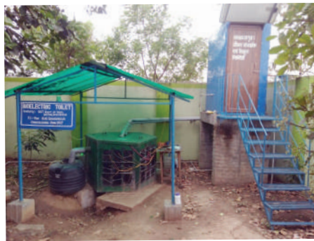
Established bioelectric toilet at IIT Kharagpur
