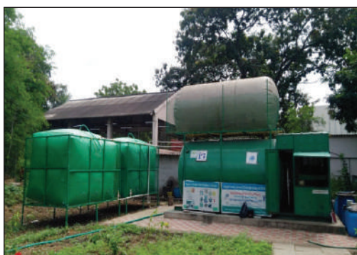
High rate Biomethanation of organic solid waste based on anaerobic gas lift reactor (AGR)
