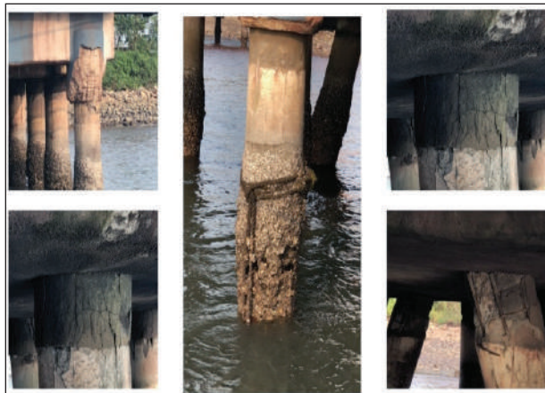
Fig. 6: Damaged Pile at berth at Paradip
