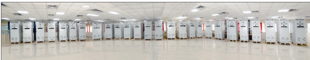
Fig.2: Power Converters shipped to FAIR
