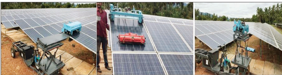
Figure 9. Photovoltaic Panel cleaning system working at solar Farm developed by PSG College of Technology
